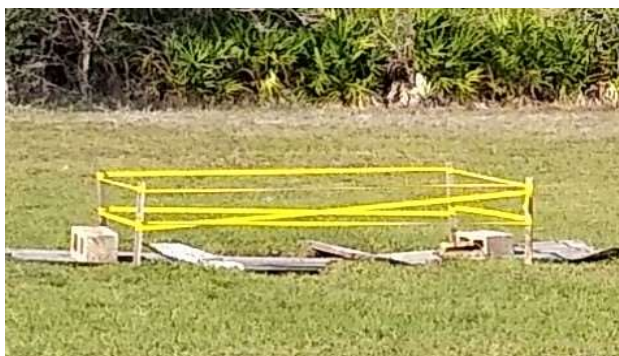
Septic tank collapsed on Indiana Drive after truck drove over it. Hopefully, the contractor rectifies this rather big oops!
